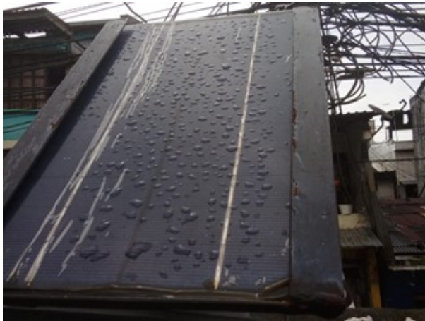
Figura 2. Panel solar instalado
